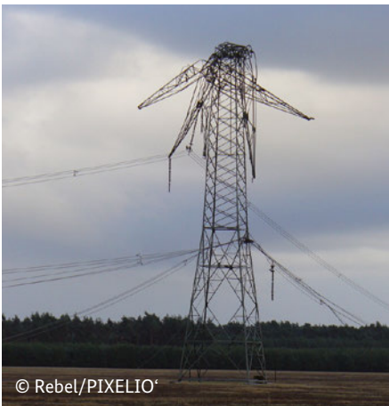
Storm damage caused by Hurricane Kyrill in 2007
